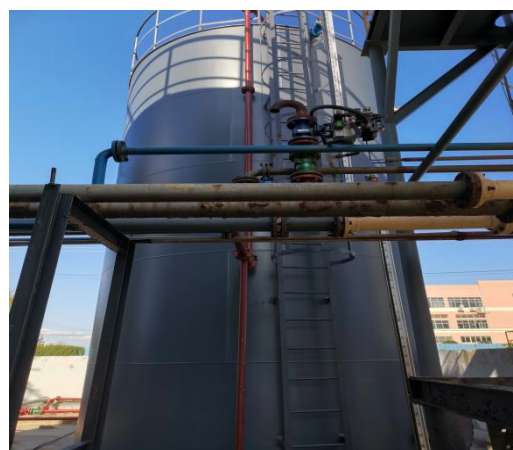
储罐自动切换阀
