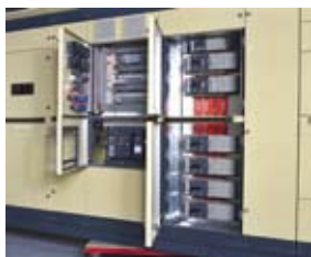
发电机组和中、低压配电 Generator Sets and Power Distribution(MV & LV)
