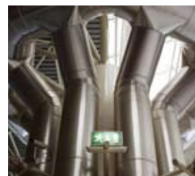
通风、空调和冷藏 HVAC(Heating,Ventilation, Air Handling & Air Condition systems) & Reefers
