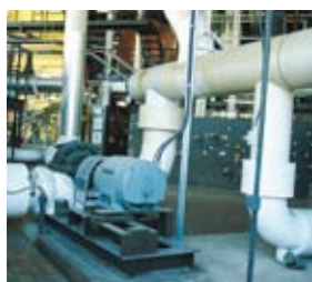
油污、水处理 Waste, Oil & Water treatment systems
