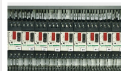
进口电器元件 Famous brand electrical parts
