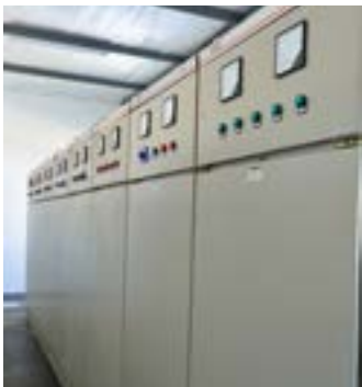
400KW/380V soft starter cabinet and control cabinet
