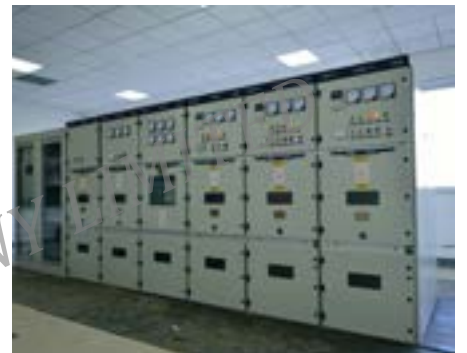
10KV Power Distribution Cabinet
